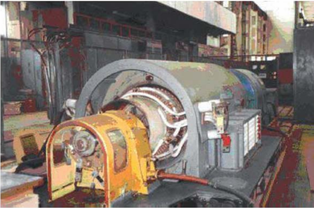
Fig. 8.30. High voltage HTS 5 MVA synchronous generator built in Russia under test [10].
